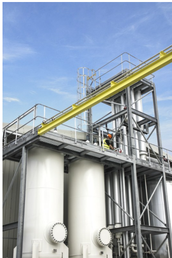
A-Gas' Refrigerant Separation Facility
